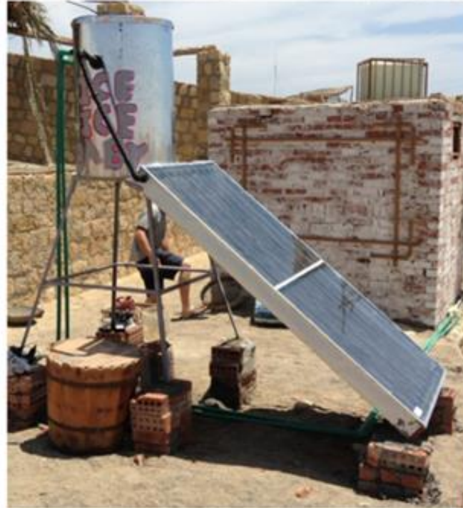
SOLAR WATER HEATER
